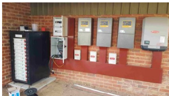
Rec Reserve battery and inverters.
